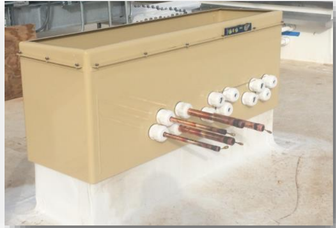
Data Center Pipe Chase Housing and Curb system (Photo shows the housing during the installation process - the lid has been removed)
