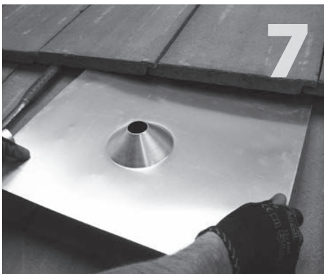
7 Cut a hole in the removed tile, with room to get the post through. Place cut tile back in position. Insert post and tighten into place. Install the 18"x 18" flashing and apply sealant around the opening.
