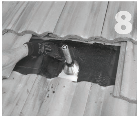
After first layer of cement is dry apply second layer over reinforcing fabric to finish waterproofing of sub-flashing.
