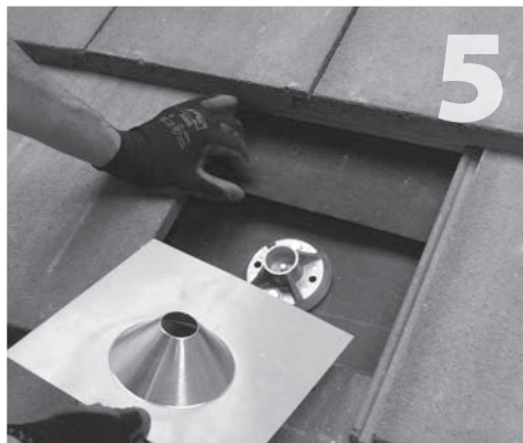
5 Carefully clean the building paper then install primary flashing in either a three-course method or properly lapped paper method.* Apply bead of sealant in the shape of an upside down U on the back side of the sub-flashing.
