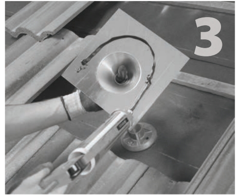
Apply a bead of sealant in the shape of an upside down U on the back side of the sub-flashing.
